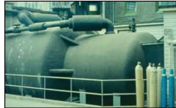
Figure 10.3: The hyperbaric chamber on the roof of the Western Infirmary, Glasgow.
